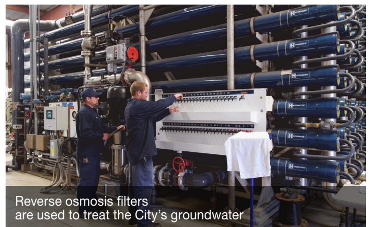
The Water Utilities Department maintains and operates the Robert A. Weese Filtration Plant 24/7
